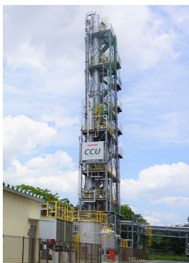
CCU facility at the waste incineration facility in Saga City
