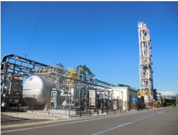
CCU at Saga City Cleaning Plant
